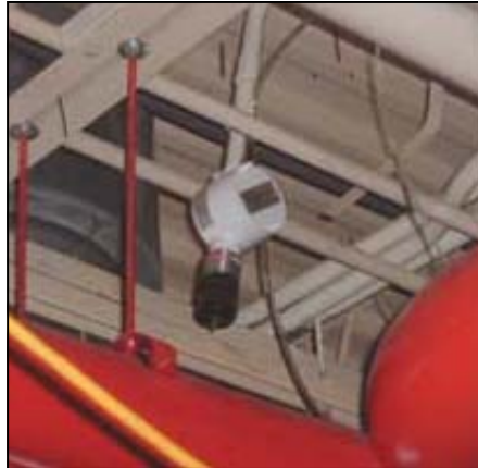
Methane sensor mounted near ceiling
